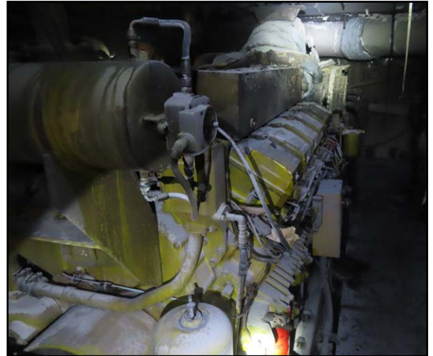
Figure 1: Damage sustained to auxiliary engine room
