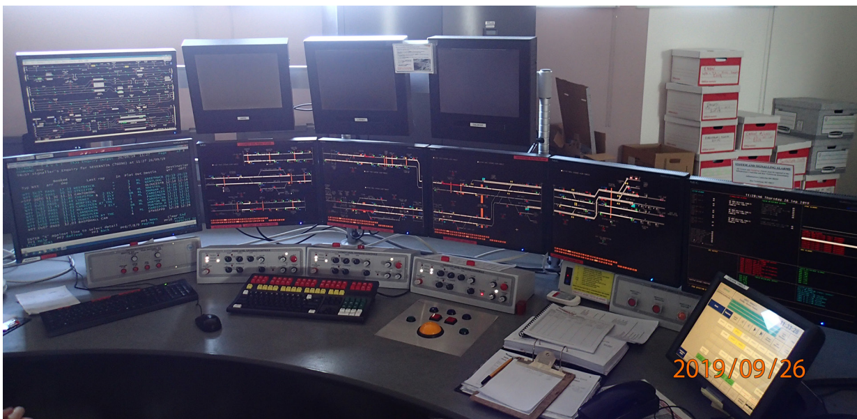
Figure 3: Example of a signalling centre with computer workstations
