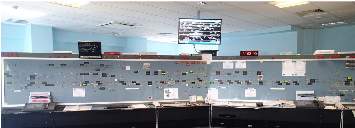
Figure 2: Example of a signalling centre with control panels
