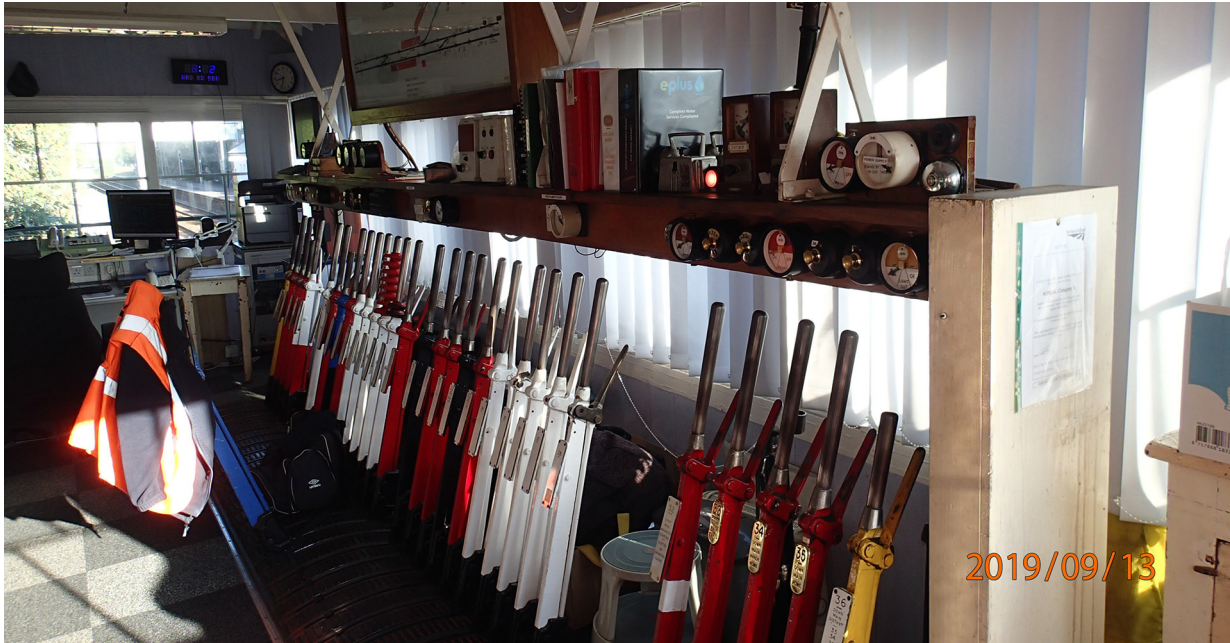
Figure 1: Example of a lever frame signal box
