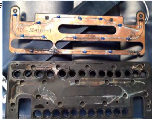
CB panel showing evidence of moisture ingress and overheating
