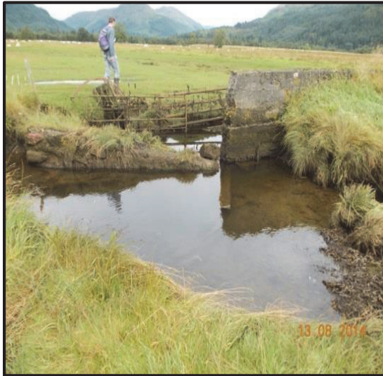
Photograph 14. Holy Loch: Earth embankment breached and failed headwall no longer functioning as coastal defence, with large expanses of low-lying grazing pasture behind.
