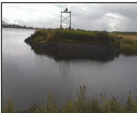
Photograph 12. Newshot Island: Towards the upstream (eastern) end of the study area the arable land and inland sewage treatment works are protected by masonry block hard engineering coastal protection.
