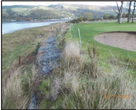
Photograph 7. Erskine South: Erskine Golf Course, with gabion baskets in a poor state of repair. The low-lying areas of the course are already subject to coastal flooding.
