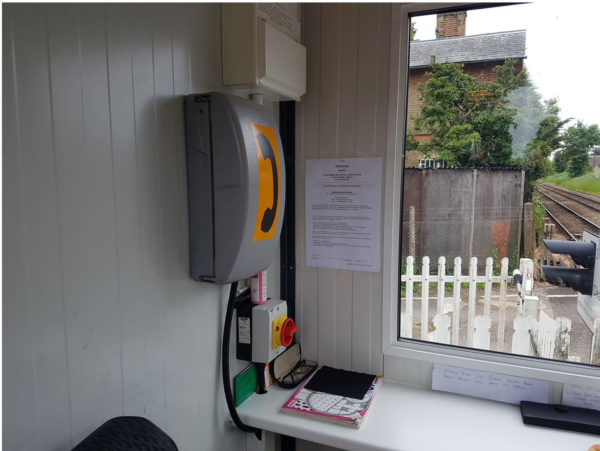
Figure 7: Crossing attendant's cabin showing gate locking switch below the telephone (installed after the incident) with view of crossing and miniature stop light equipment.
