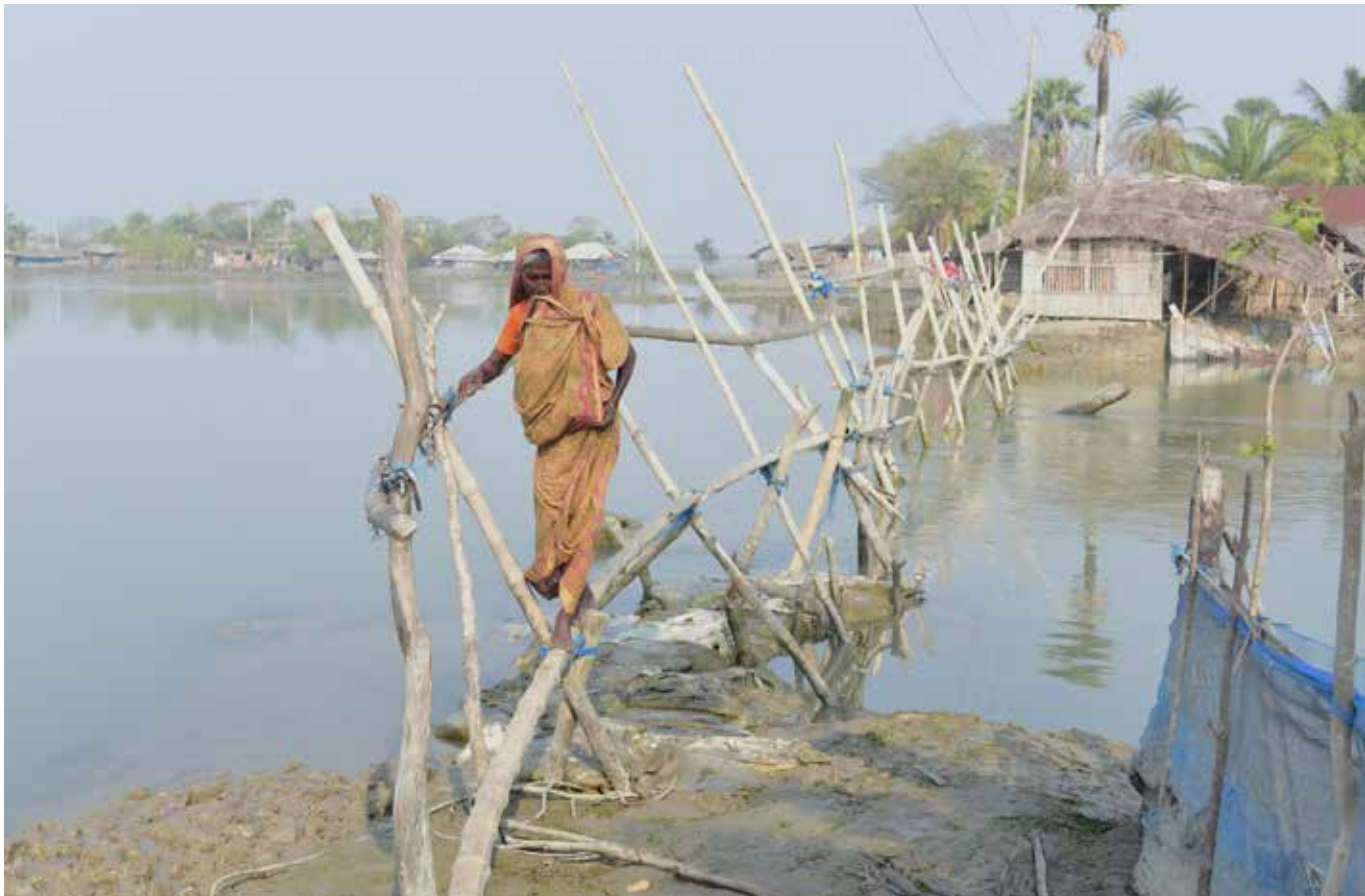
Roads and Infrastructure damage Bangladesh, credit Shahin Alom
